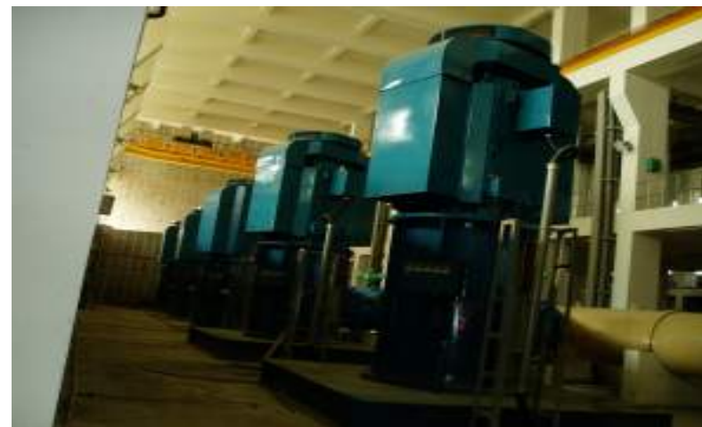
4000HP 10P 6.6kV 60Hz VSS TEAAC Motors for Taiwan Water Co. Suction Pumps
