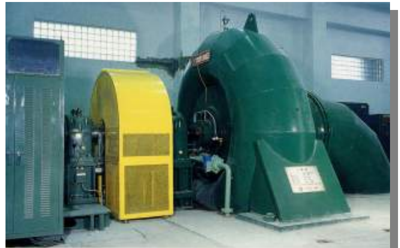
Kao-Pin Hydraulic Power Plant, 2,250kW 18P 2sets
