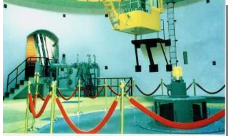
Sui-Lien Hydraulic Power Plant, 9,500kW 10P
