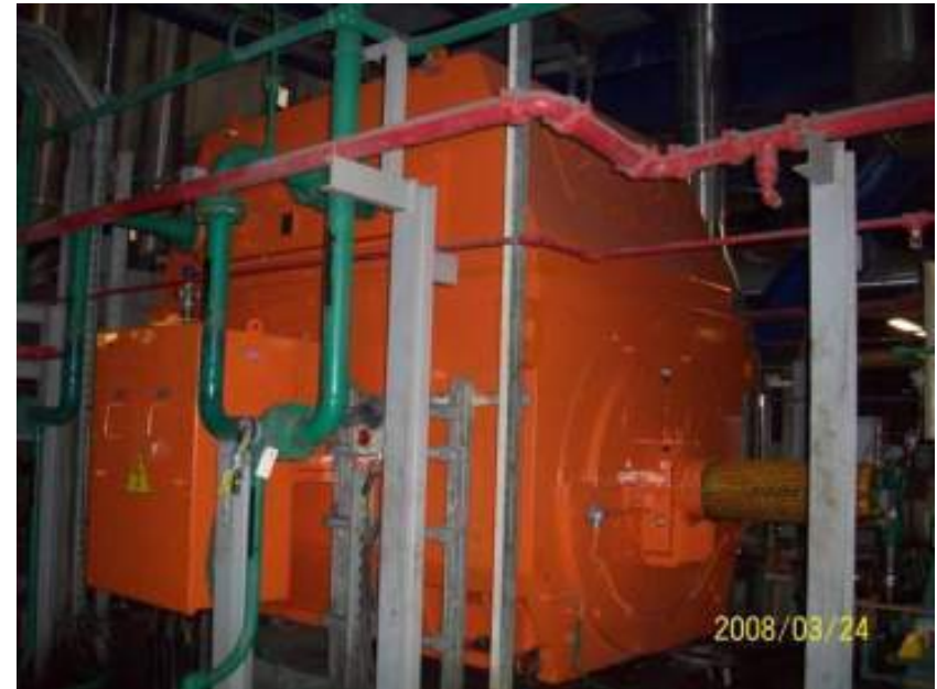
10,330kW 4P 13.2kV 60Hz TEWAC Motor for Boiler Feed Pump Application at Power Plant
