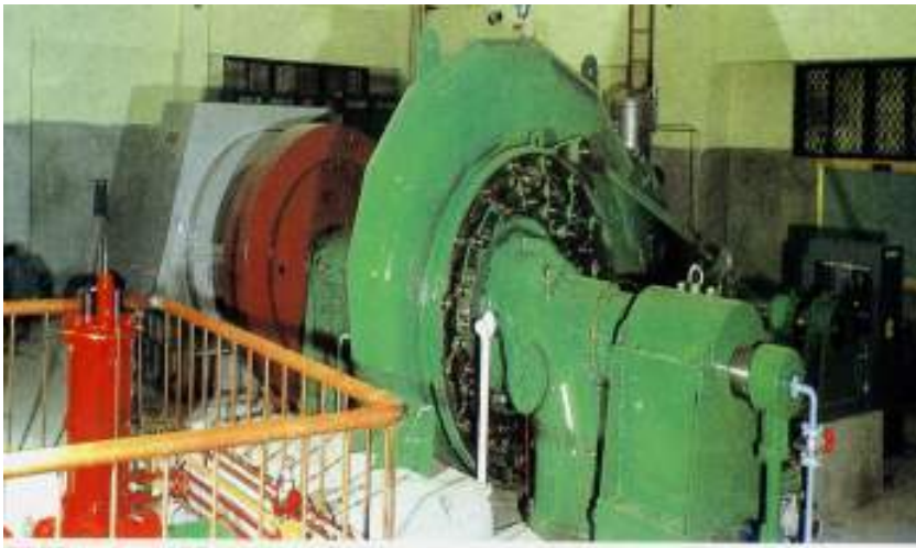
Ching-Liu Hydraulic Power Plant, 4,200kW 12P
