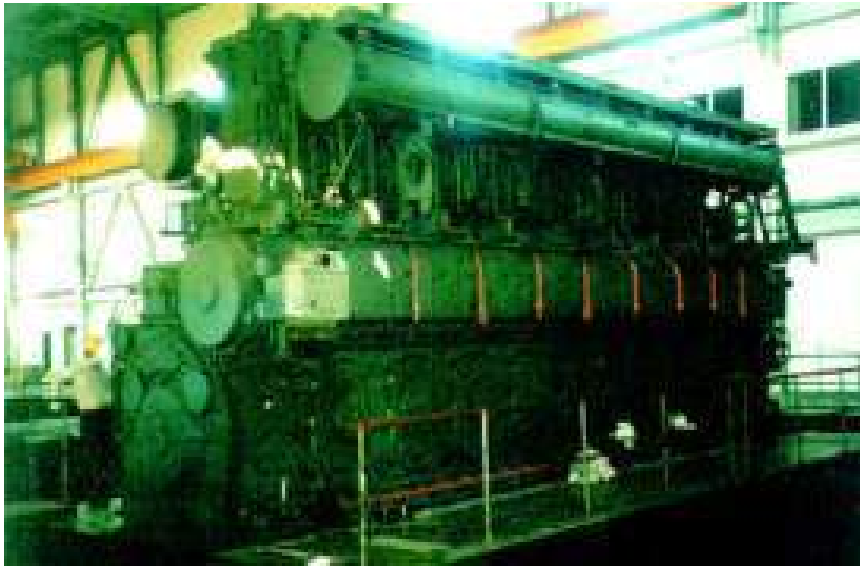
(Peng-Hu 2nd Power Plant 10,000kW Diesel Engine Generator System)
