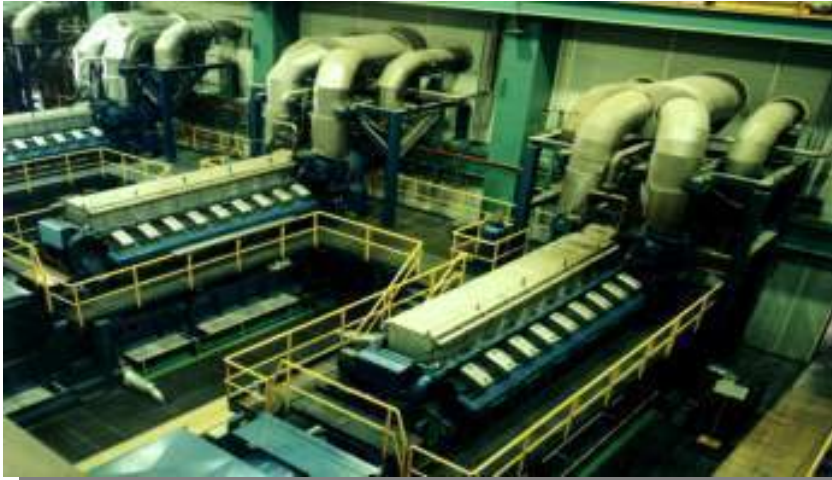
C.P.T. Cogeneration System, 6,300kW 10P 4sets
